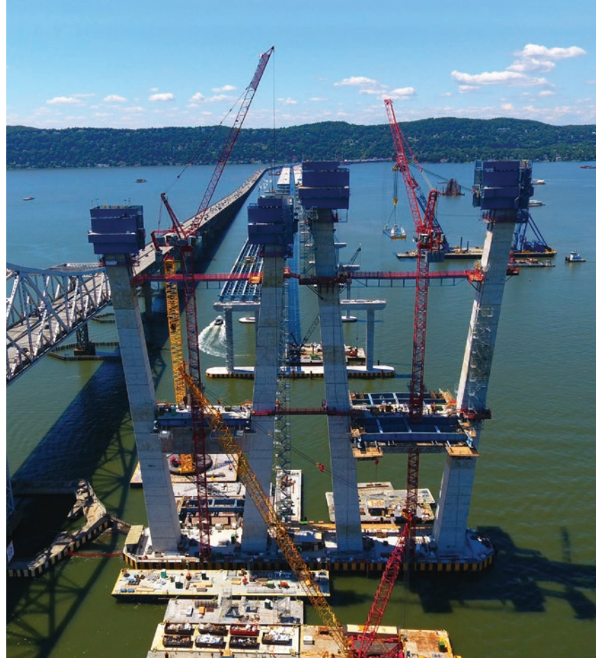
Self-climbing jump forms were used to build the iconic main span towers.
