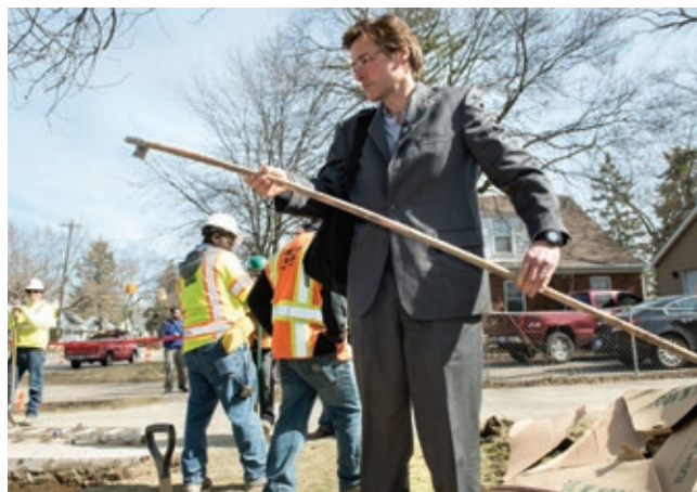
Edwards examines a length of pipe that supplied the home of Flint resident Elnora Carthan.
